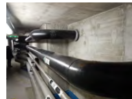
Picture of a section of SEK piping in the gallery
