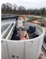
Assembly of lamellar modules during the visit to the Laon's water treatment plant
