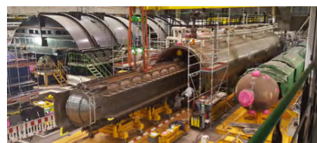
Extraction of a bundle from the GSS shell
