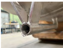
Piquage having undergone a rupture by vibratory phenomenon
